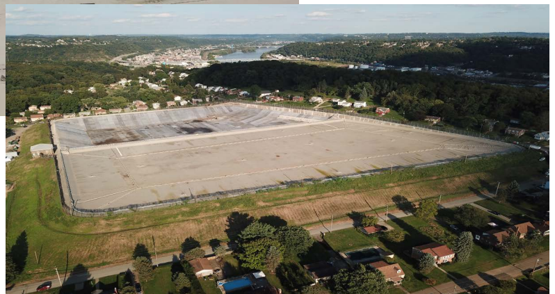
The West Cell of Lanpher Reservoir completed with the East Cell still under renovation. The storage facility serves one-third of PWSA's customers.
