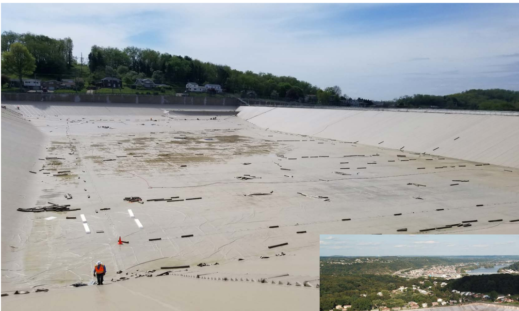
Crews work to replace the cover on the East Cell of the Lanpher Reservoir.
